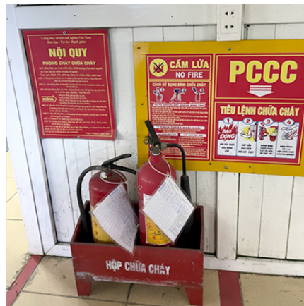
Fire extinguishers, inspected periodically
