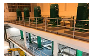
Lusail sewage treatment plant
