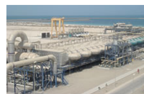
Taweelah B Power & Desalination Complex
