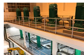
Lusail sewage treatment plant
