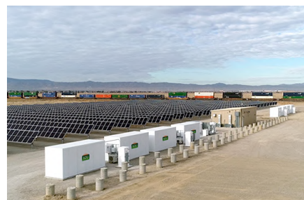
Energy storage facility using EV batteries
