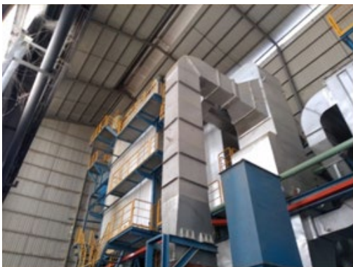
▲ Bubbling fluidized bed boiler
